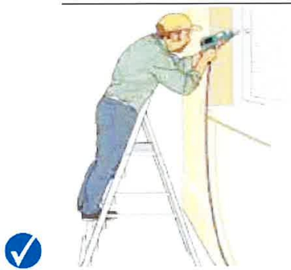
Correct – steps facing work activity
